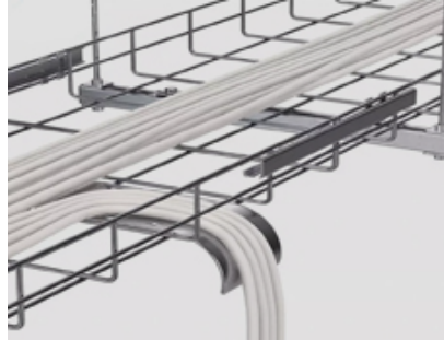
Grid Bridge / Metal Mesh Cable Bridge
